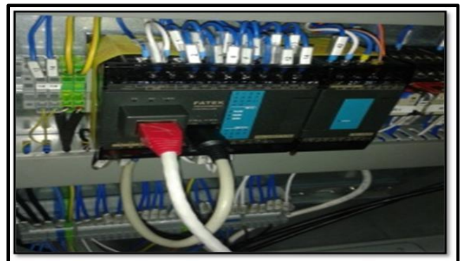
Fig. 8 PLC control unit
