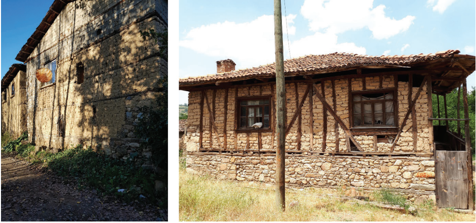
F. 9: An adobe masonry ground floor in Kusumlar village (Güneş Kaya, 2019) and a stone masonry ground floor in Sadağı village (Güneş Kaya, 2018)
