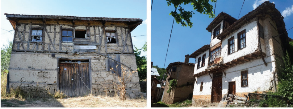
F. 5: A two-story house from Süleymanbey village (Güneş Kaya, 2019) and a three-story house from Dağgüney village (Güneş Kaya, 2017).
