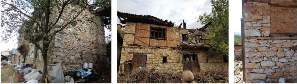
F. 10: Stone masonry walls that continue on the upper floor in Serçeler village (Güneş Kaya, 2018 and 2020) and detail of a continuous stone masonry wall (Güneş Kaya, 2018)
