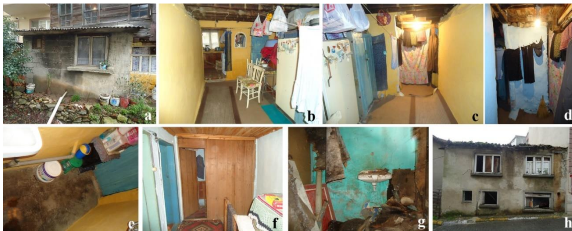
Figure 7. Photographs of elements with deteriorations and corruptions
