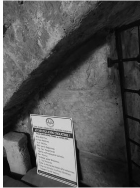
Fig. 5 Inside View of the Vault from the Upstream Side (Photo: İlkay Göçmen).
