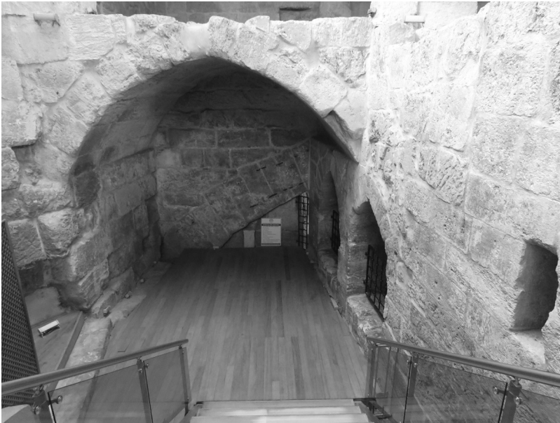
Fig. 6 Archivolt and the Spandrel Wall of the Upstream Façade (Photo: İlkay Göçmen).
