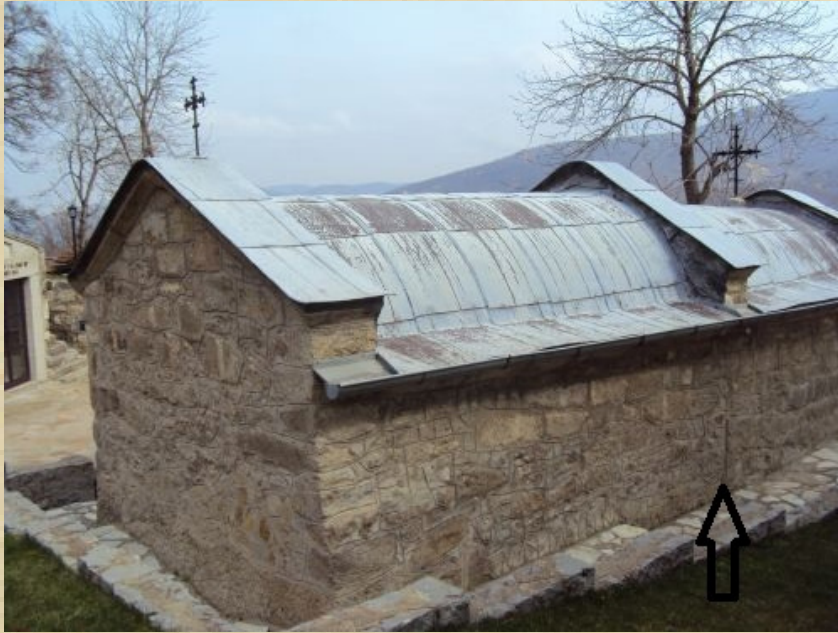
Fig. 2. The church from the back, the point where the arrow points is the meeting of the new building from the old one. photo author
