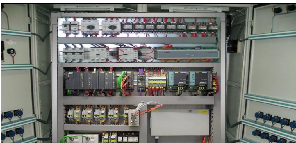
Figure 7. Created power transformers faults detection panel
