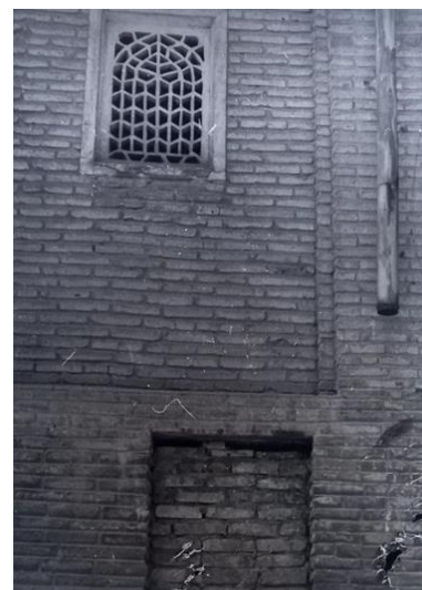
Figure 15. The entrance of the Chilakhana in an old photo. It was closed at the last restoration study (Madaniy Meros Agentligi, 2022)
