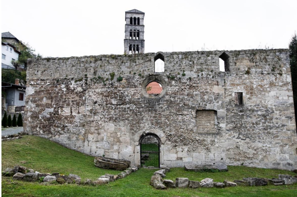
Figure 6. Jajce, church of St. Mary with the tower of St. Luke (photo Mario Periša, 2019)
