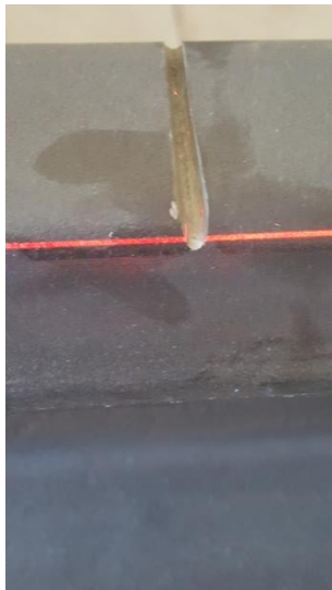
c) crack rail line
