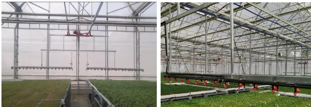
Figure 11. The new rail-type irrigation system
