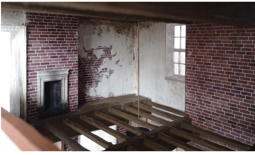
Figure 33. County House, model of café. Where areas of structural damage are severe, it would be against the principles of incidental narrativity to inconspicuously restore these spaces. Instead, stabilization works will take place, denoted using brass columns, while the removal of rotten floorboards allows lighting, signage and museum displays to be hung through the remaining joists. Changing levels within the building are resolved by building up the floor height in new timber walkways, with lower levels becoming display areas.
