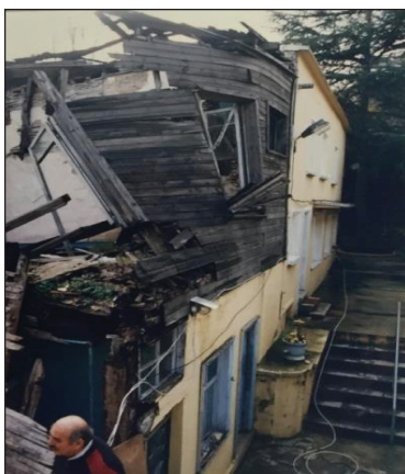
Photograph 27. It is a Mamigonyan School in Ruins (preservation board archive).
