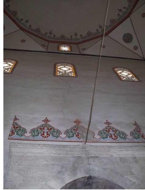
Fig. 7 Crack on the B3B6 wall
