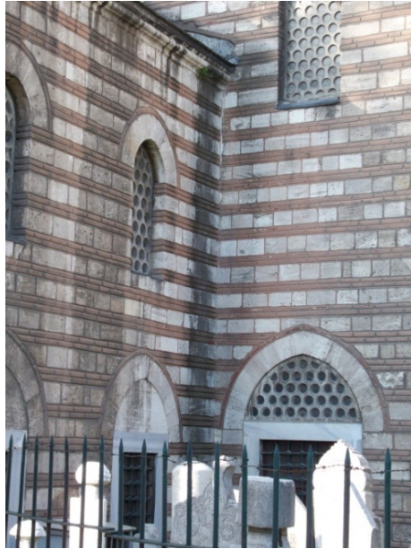
Fig. 9 The corner joint of the walls of adjacent part and main part of the building
