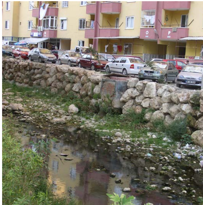
Figure 7. The sewage drainage to the watercourse in the area.
