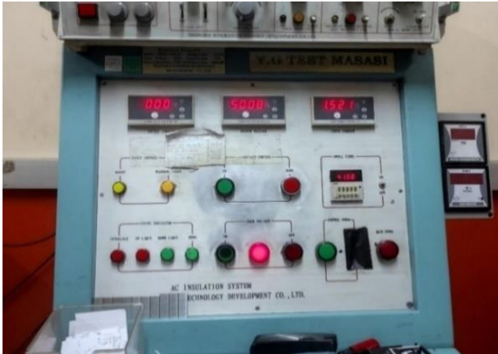
Figure 5. Insulation test image of the transformer below 50 kV
