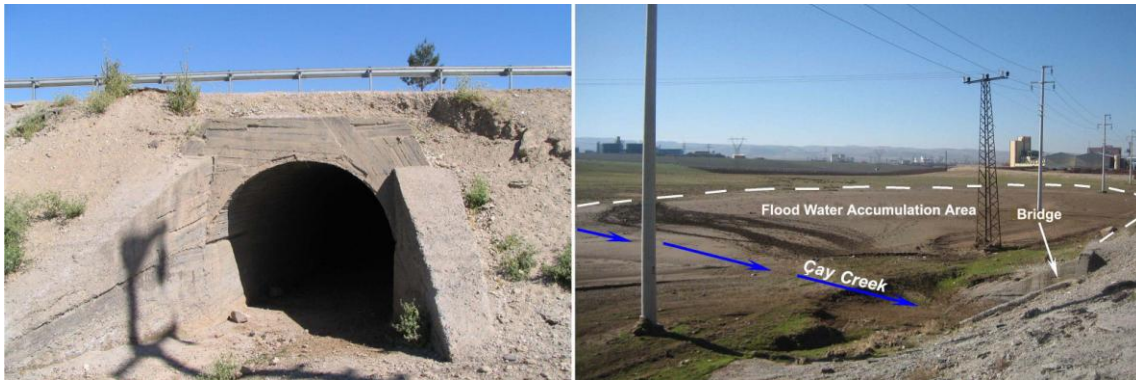
Photo 9. Bridge over Çay creek at entrance of Batman city and areas where water accumulates in times of flood.
