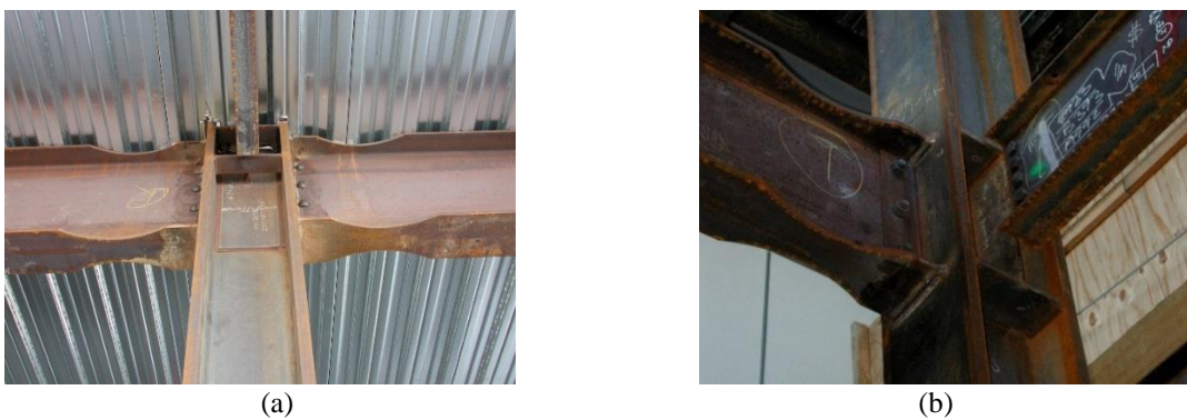
Figure 14 Column Bracing Samples: (a) Bracing at the Top Flange, (b) Bracing at the Top and Bottom Flange
