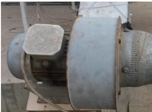
Figure 10. Motor and fan of the SAH.
