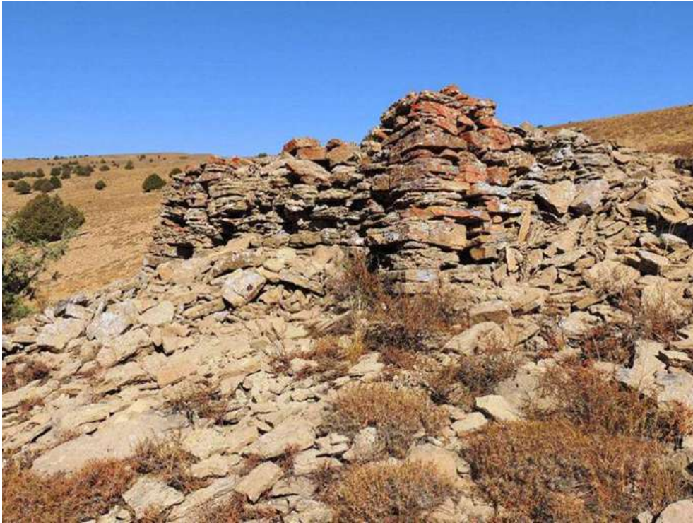
Fig. 39 Destroyed facade of a construction.
