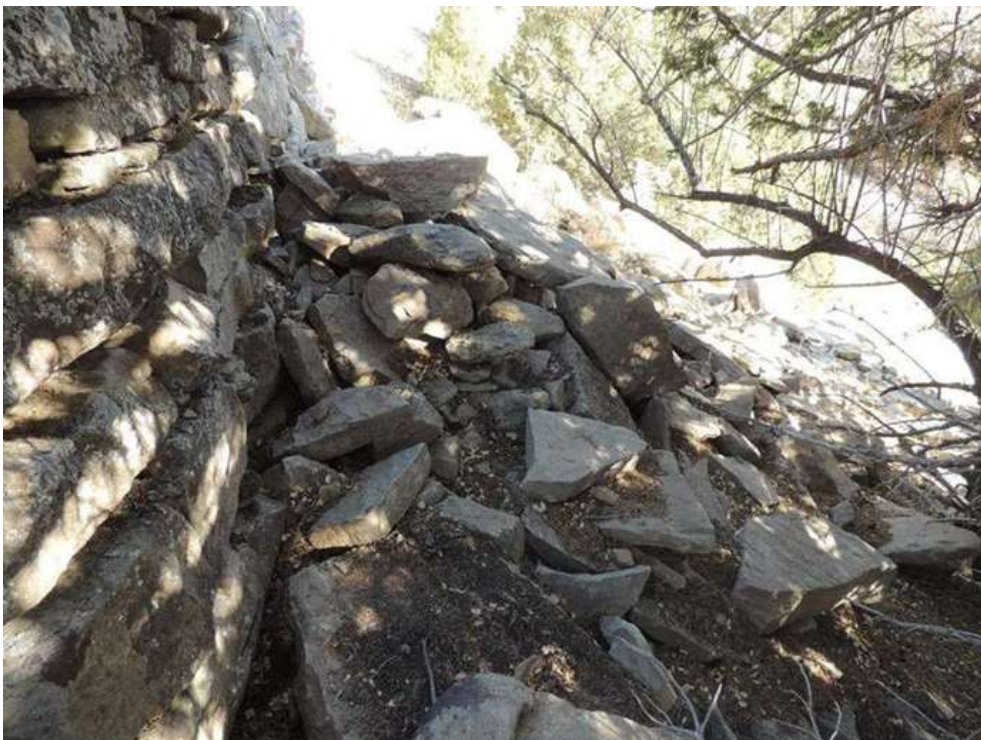
Fig. 36 Base of construction 13 with fallen block of stones.
