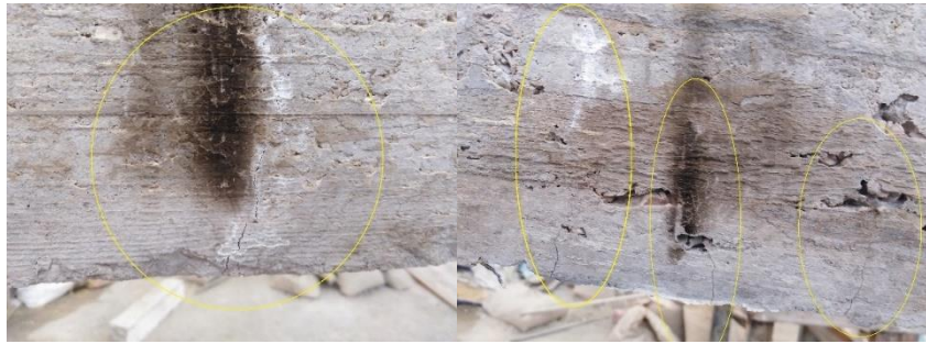
Figure 27. Expansion of the crack's width
