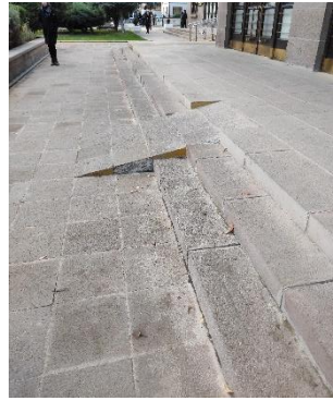
Figure 8. Stairs and ramps without handrail ( A51, A54, A76, A81, A88)
