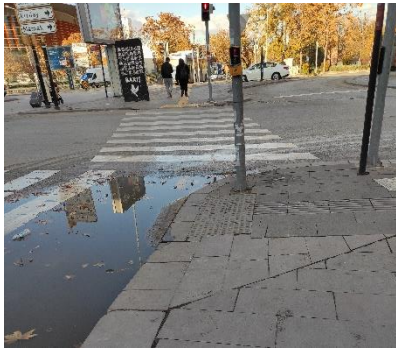
Figure 7. Drainage problem (A145)
