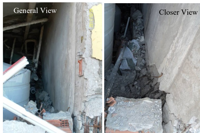
Figure 8. Separation of shear wall SW4 from the foundation (A4-B4).
