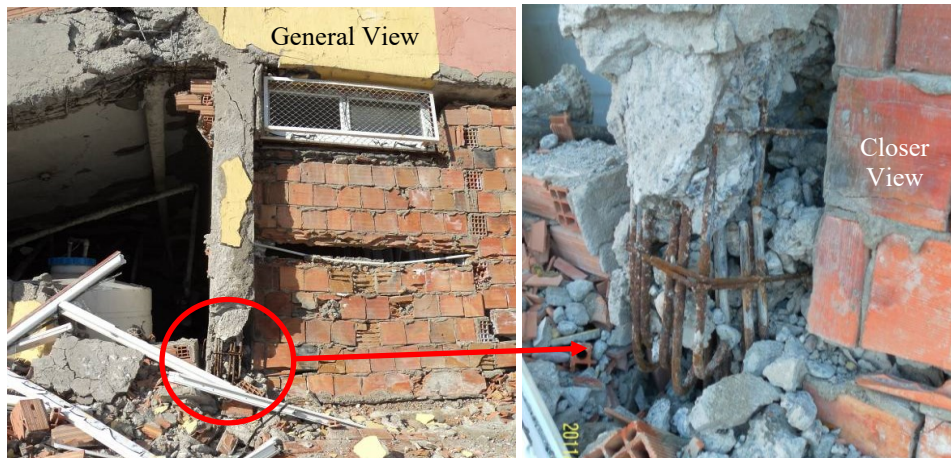
Figure 7. Failure of shear wall SW4 (A4-B4).
