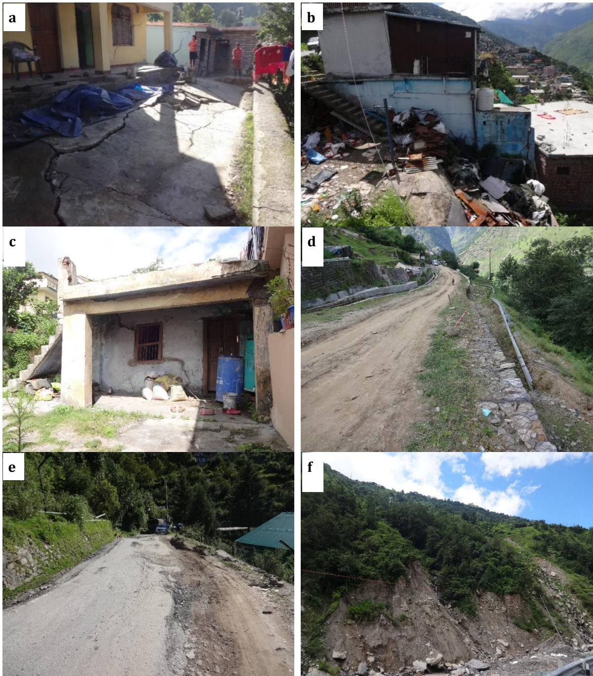
Figure 5. Damage to property and infrastructure due to land subsidence events; (a) Wider cracks in walls of houses and courtyard at Sunil village, (b) detached column of a house at Gandhinagar, (c) transverse cracks on the wall of a house at Ravigram village, (d) road subsided just below NTPC colony near Marwari area, (e) a water supply line was observed to be dislocated caused road subsided in the Sunil village, and (f) severe toe erosion by Alaknanda river on its left bank
