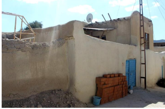
Foto 2e. Ali Şen evi kuzey cephe (Photo 2e. Ali Sen house the north front)
