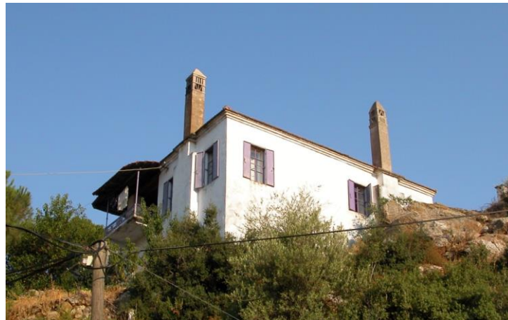
Figure 25. It is seen that the stone facade walls of many residential buildings have been plastered with cement-based plasters and have lost their original appearance (photo belongs to the author)
