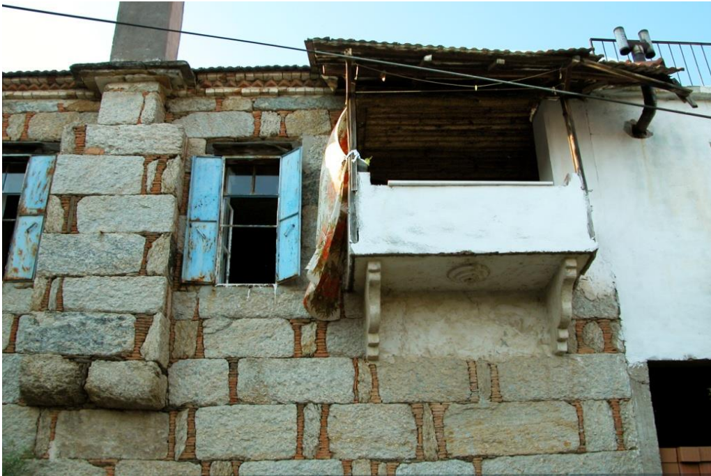
Figure 27. Many of village houses have lost their original features as a result of additions and alterations with inappropriate methods and materials (photo belongs to the author)
