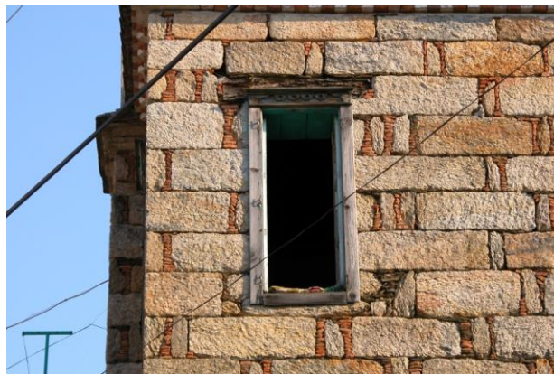
Figure 10. An example of stone masonry from Çomakdağ / Kızılağaç house (photo belongs to the author)
