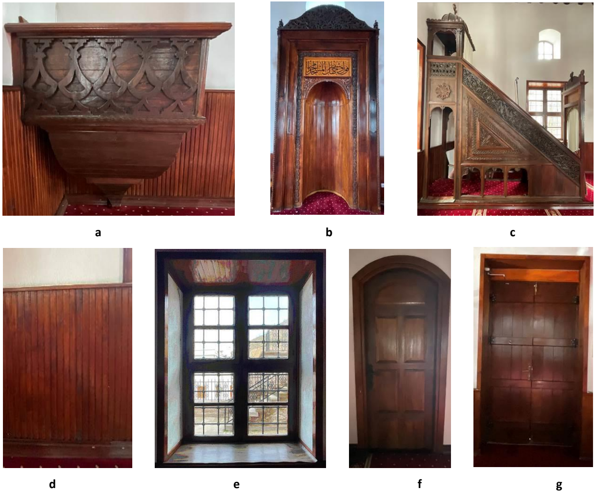
Figure 14a-b-c-d-e-f-g. Examples of places where wood is used in Sille Çay Mosque
