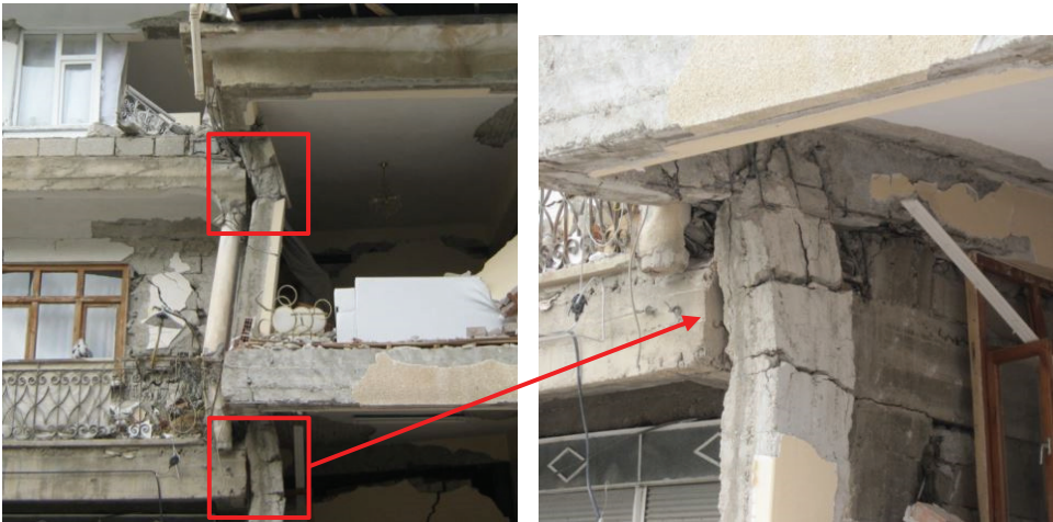
Fig. 1 – Examples of Pounding failures. [13]
