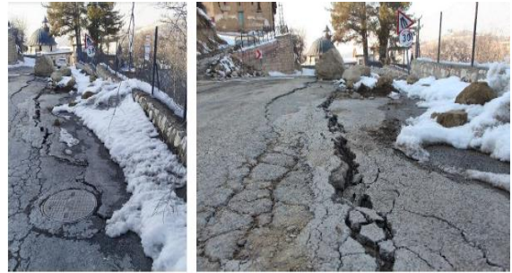
Figure 30. The asphalt pavement cracks due to the lateral movement of retaining wall in Yeşilyurt district
