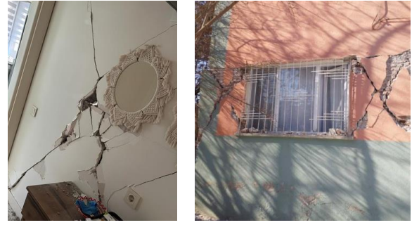
Figure 22. Shear cracks in walls
