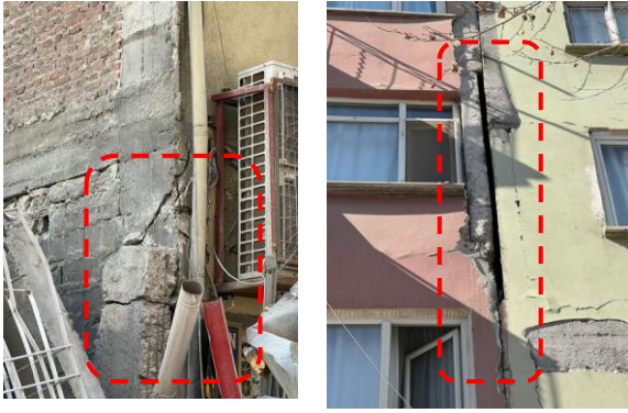
Figure 12. Pounding effect in adjacent reinforced concrete buildings caused by the lack of seismic gap
