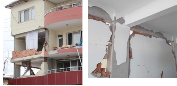
Figure 23. Out-of-plane toppling of walls and frame-wall separations
