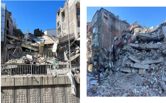
Figure 10. Totally collapsed buildings in Malatya
