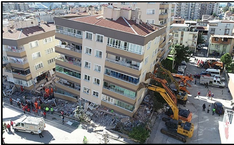
Şekil 12: Deprem sonucu aldığı hasar (BBC News Türkçe 2020) Figure 12: Damage as a result of the earthquake (BBC News Turkish 2020)
