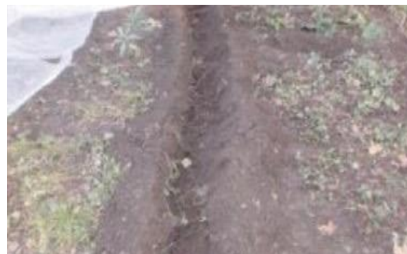
Figure 6. Excavation for undergrounding the wire mesh used to cover the root system of Platanus spp.
