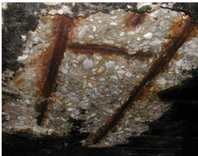
Fig. 1 Corrosion damage at Güllük pier (Baradan et al., 2013)
