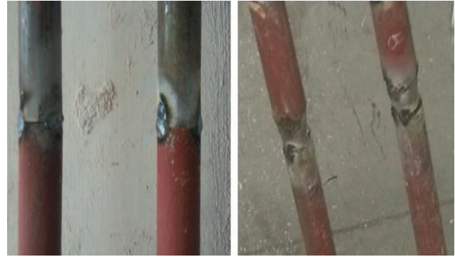
Figure 2. Application example of pipe welding fault (C3).
