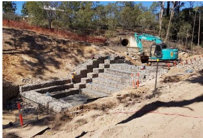
Figure 9. An example of full protection of a culvert outlet downstream with natural materials
