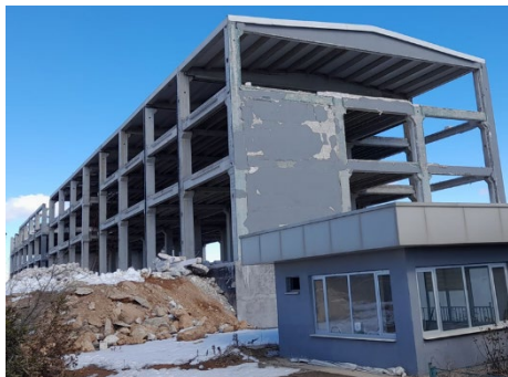
Şekil 6: Deprem hasarı almış 3 katlı betonarme prefabrik yapı Figure 6: 3-storey reinforced concrete prefabricated building damaged by earthquake
