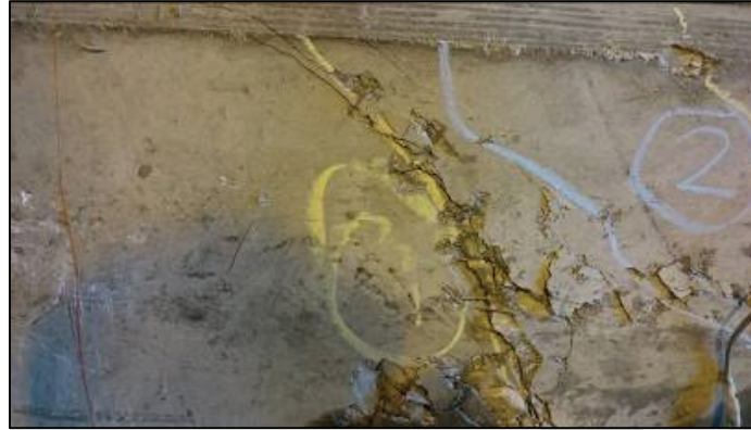
Figure 10 - SFs prevent the cracks
