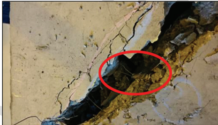
Figure 11 - The rupture of transverse reinforcement (S30V09 beam)
