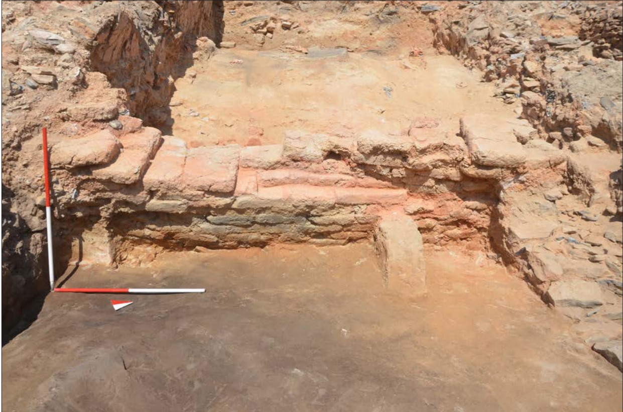
Figure 4. Seyitomer Hoyuk Phase V/D, Room 82, mud brick partition / Seyitömer Höyük V/D evresi 82 no'lu mekan, kerpiç ara duvar.
