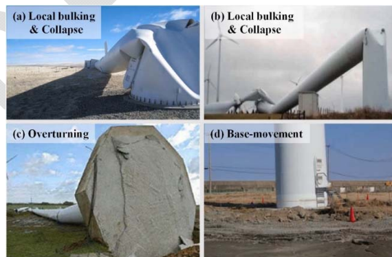
Figure 2 - Possible damaged of WPP due to earthquake (REF)
