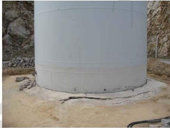
Figure 1 - Damage at the connection of the tower and the foundation of the WPP
