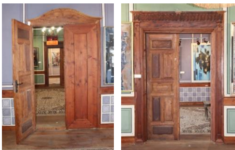
Fig. 30. Front and back views of the door in Stombalyan house (Şahin H. 2021).
