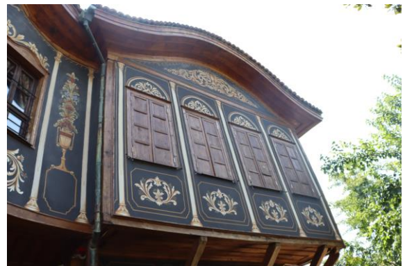
Fig. 16. Bay window and the vault-like structure formed by a three-centered arch in Argir Kuyumcuoğlu house (Şahin H. 2021)
