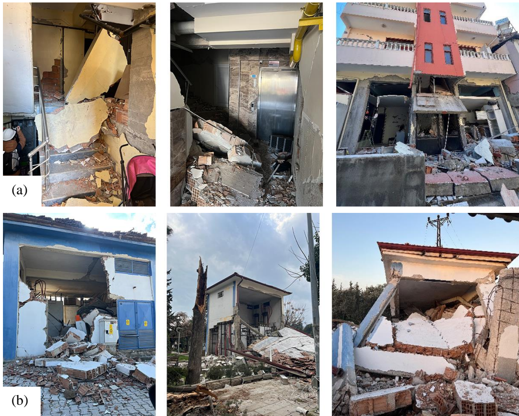
Figure 3. (a) The closing of the building exits with the overturning of the infill walls, and (b) the infill walls in the energy transformers being inoperative by overturning after the Kahramanmaraş earthquakes
