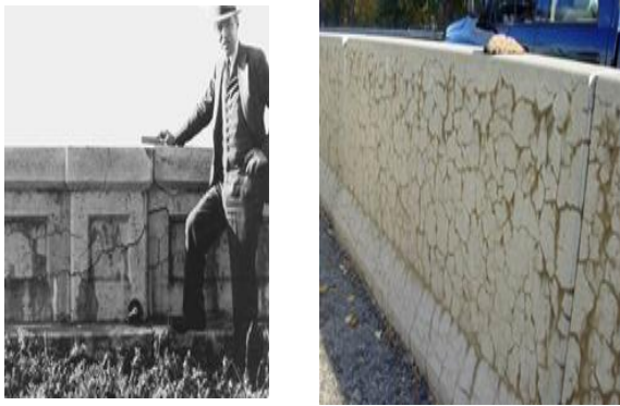
a- Alkali silica reaction cracks and Thomas E. Stanton (Photo extracted from California Department of Transportation)
