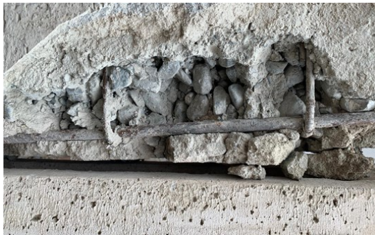
Figure 17. It is seen that the concrete was placed with segregation and without a vibrator.
