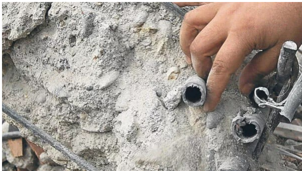
Figure 13. Shows manual crushing of concrete to indicate poor concrete quality.
