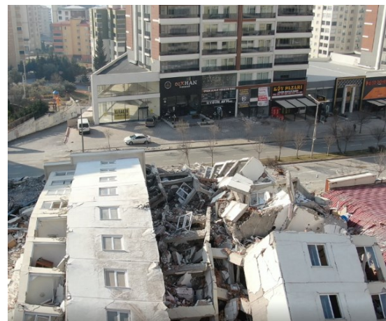
Figure 20. Kahraman Maraş onikişubat haydar bey mah. The building collapsed due to column cutting.
