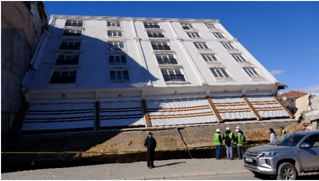
Figure 2. A building that moves vertically due to soil liquefaction - sand boiling but remains intact with its elements.
