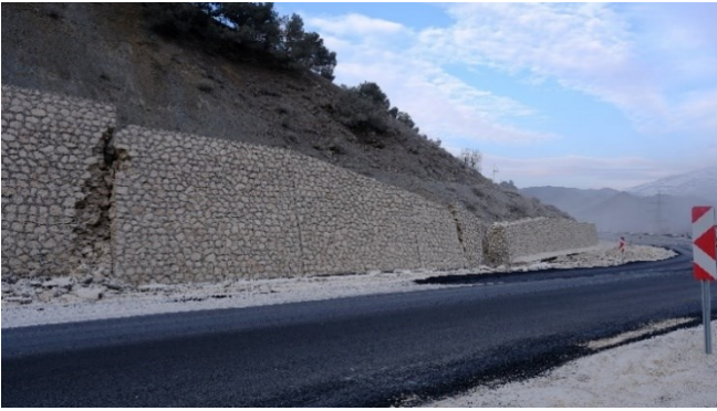
Figure 9. Examples of damage to the structural stone walls
