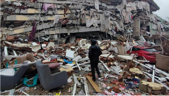
Figure 6. A collapsed building in the Malatya Özalper Neighborhood collapsed due to a weak column-strong beam.
