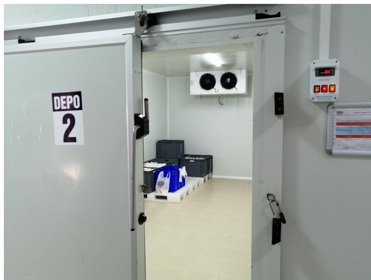
Figure 3. Image of the Burdur Mehmet Akif Ersoy University Dairy Products and Technologies Application and Research Center, Dairy Factory, Final Product Storage Room.
