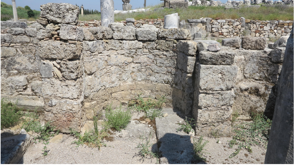
F. 26: The apse of the Small Church, view from the west (A. Tiryaki, 2022)
