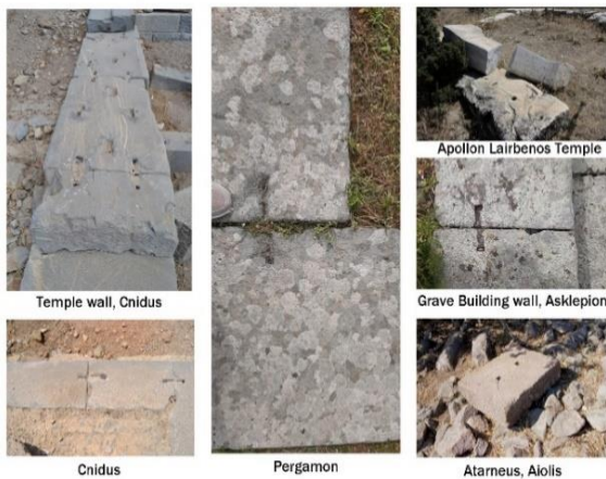
Figure 3. Traces of clamps and dowels in different ancient Anatolian cities (photos taken by the author in 2024)
