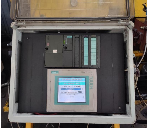
Figure 5. Automation part of the experimental setup installed with S7-300 PLC
