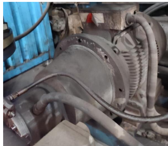
Figure 1. Pump and the electric motor powering the pump
