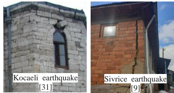
Figure 1. Continue Damage situations of masonry structures
