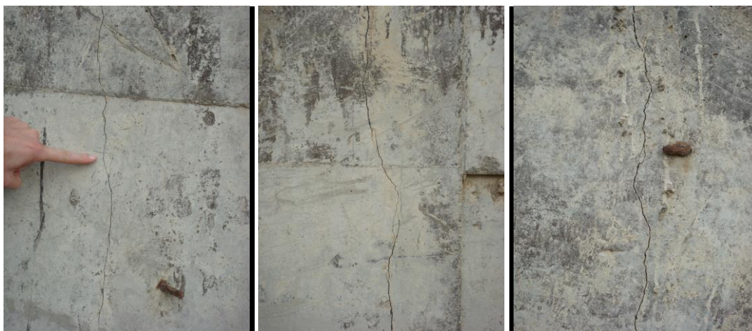
Figure 9. Concrete cracking in foundations due to collapse settlements
