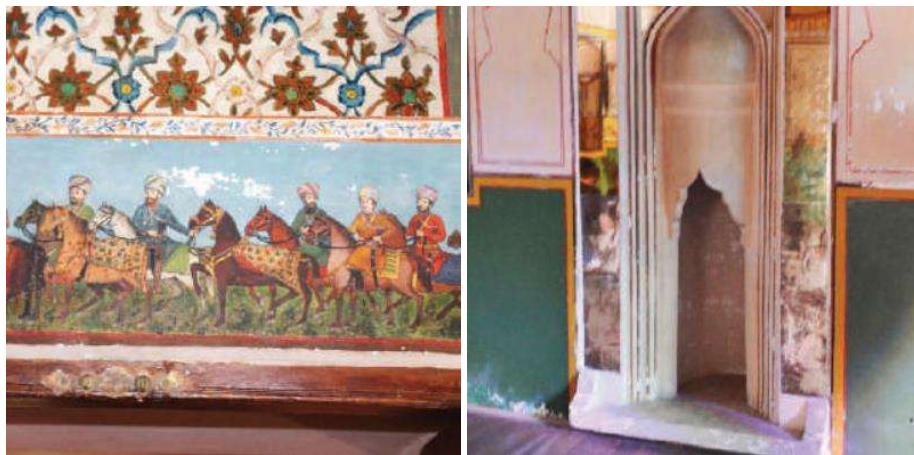
Figure 10. Cracks and deteriorations in some paintings in the Sheki Khan Palace.
