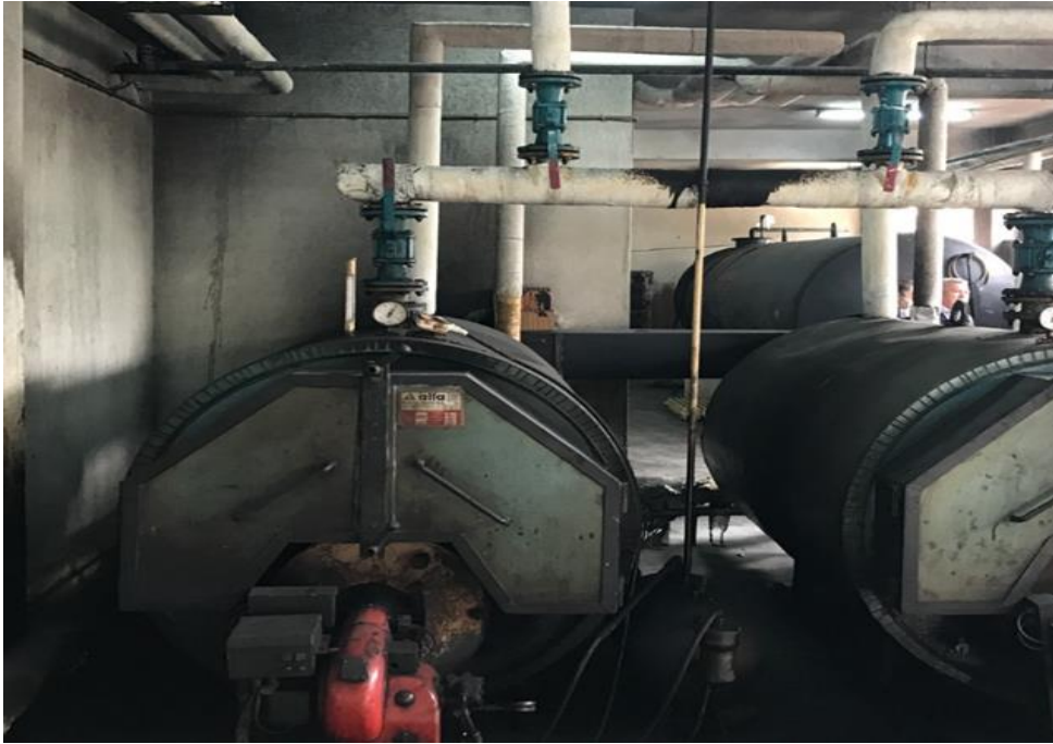
Figure 3. Old Heating System Boiler and Burner Collector Images
