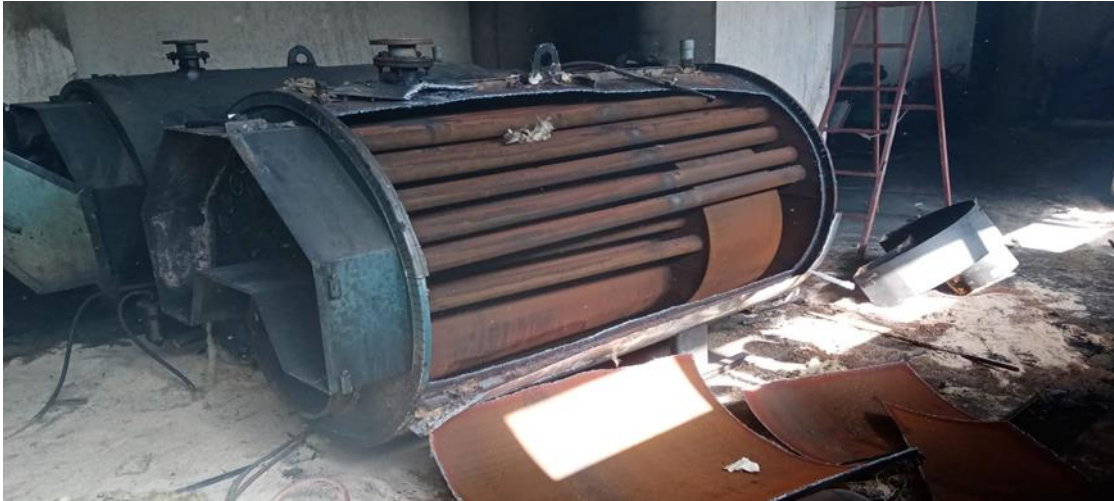
Figure 2. Old Heating System Images
