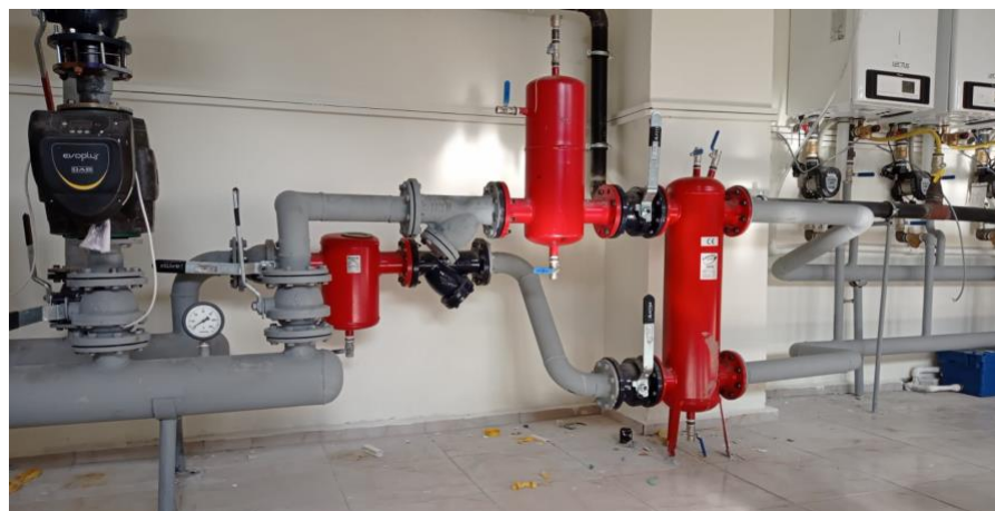
Figure 7. Cascade heating system pumps and balance tank installation
