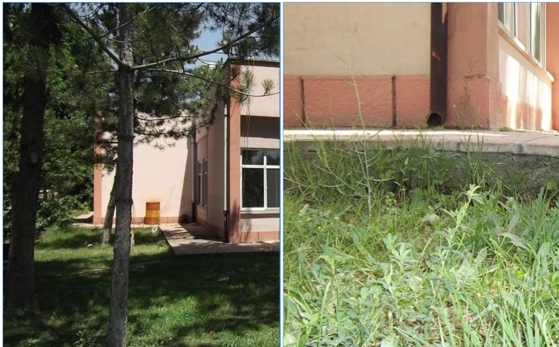
Fig. 7. Photographs showing rain gutters discharging into the pavement
