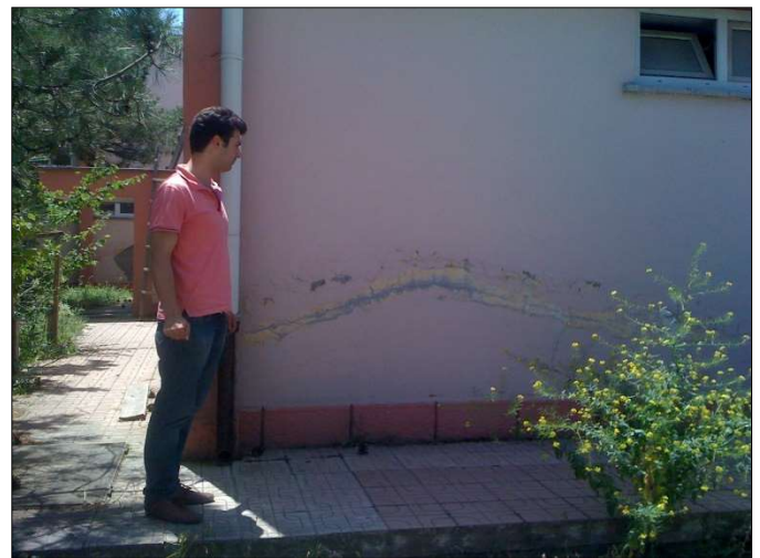
Fig. 4. Stucco blistering on the north side of the building
