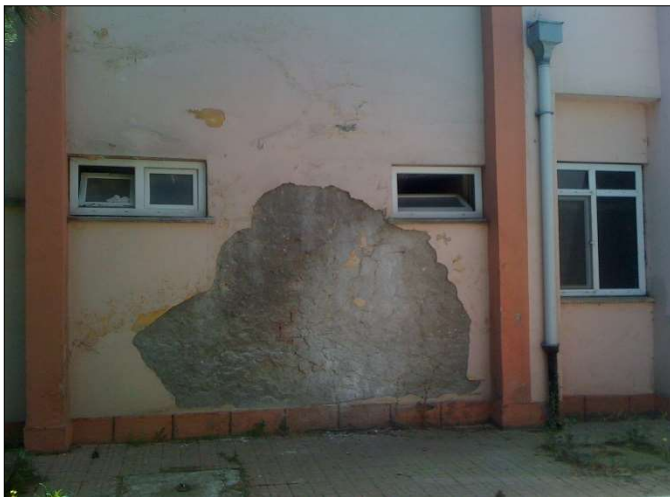
Fig. 3. Plaster spills on the east side of the building
