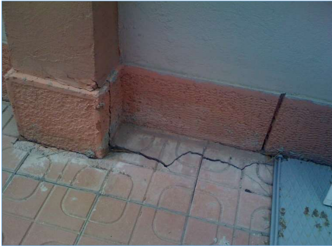
Fig. 5. Floor and wall cracks on the west side of the building
