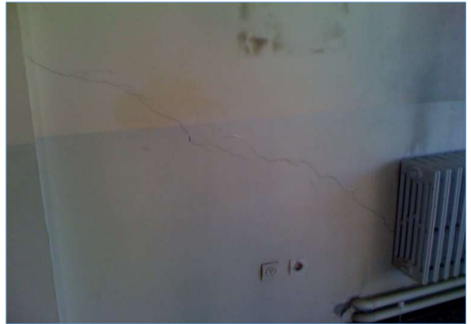
Fig. 6. Wall crack inside the building
